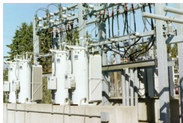
5 kV Voltage Regulators
