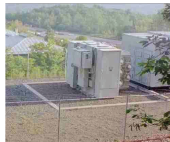
Transformer with Automatic Load Tap Changer
