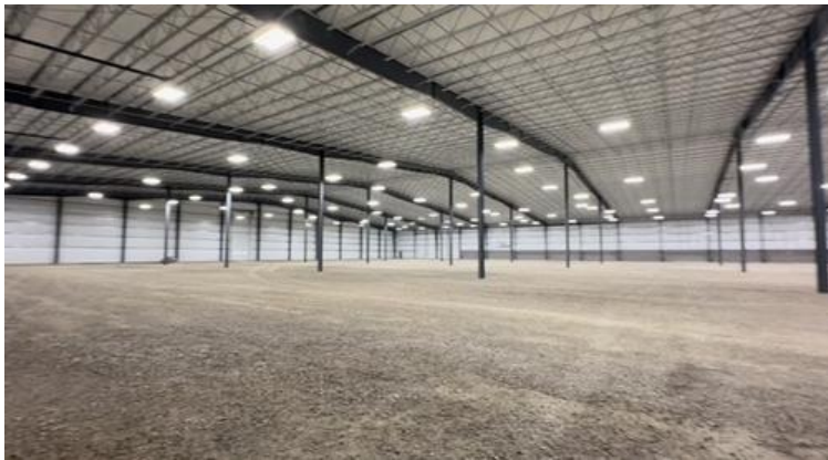
Spec 10 Inside Photo
